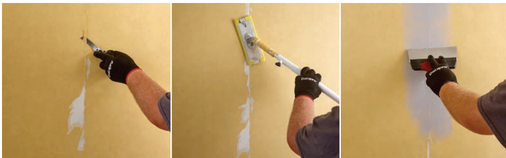
Start by removing wallpaper that has come loose. Then apply filler to all cavities, cracks and wallpaper joints. Fine smooth structured wallpaper or severely damaged surfaces one or two times.
